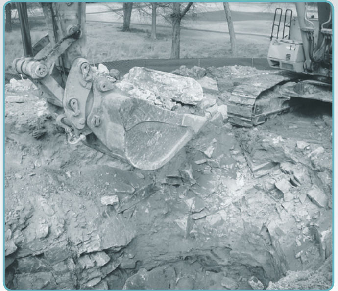
Crews excavate rock on the Charlotte Country Club property in preparation for pipe installation.
