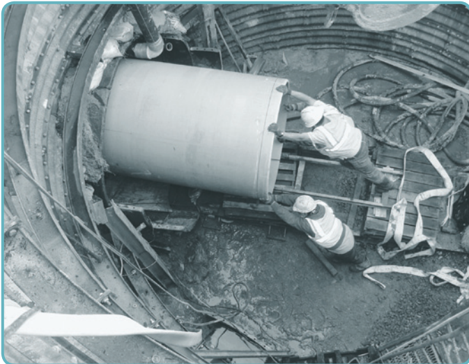
Tunneling crew push carrier pipe into the tunnel under 7th Street/Monroe Road.
