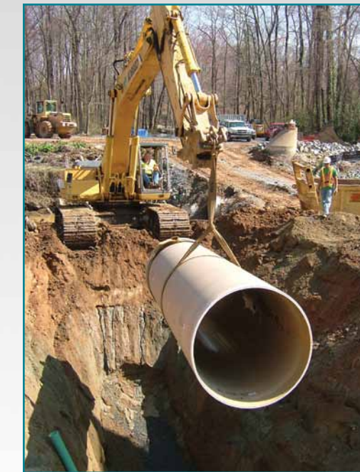
Crews install a section of pipe near Meadowbrook Drive during Phase I of construction.
