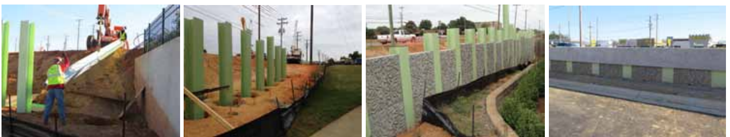
Pre-cast concrete panels are placed between steel H-piles creating a decorative wall.
