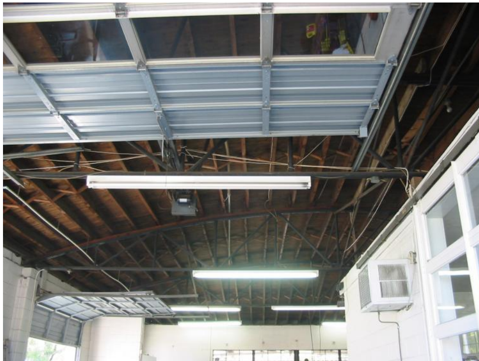
Plate 71. Elmore Trailer Sales and Trailer Park, Sales and Service Building, Interior, Service Area.
