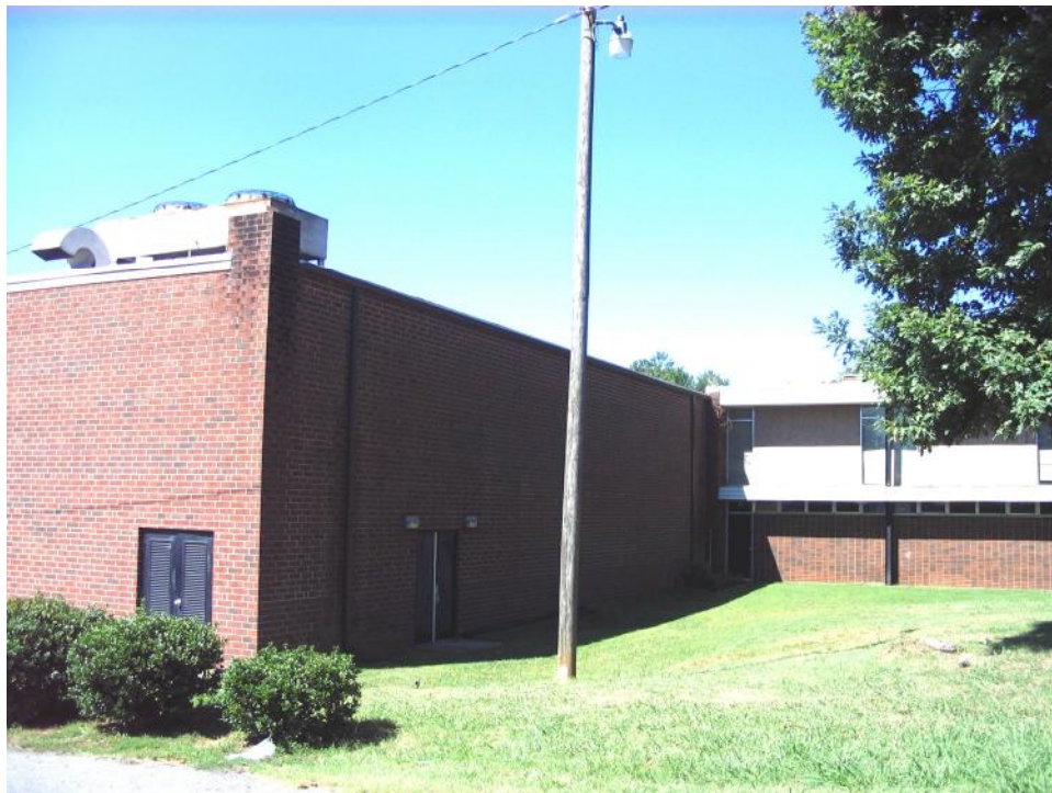
Truck Drivers Union (AFL No. 71) Hall (No. 76), Auditorium Addition, North and East Elevations, Looking West.
