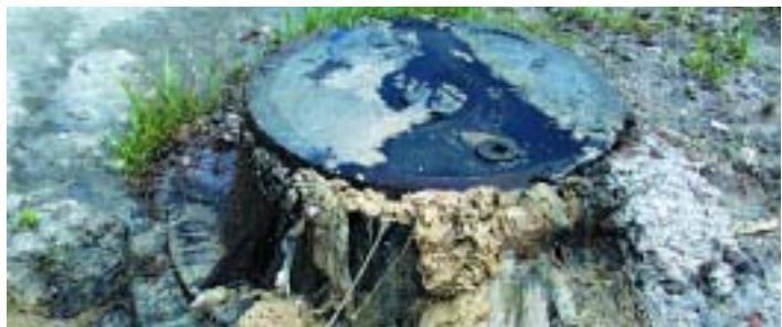
Cooking grease poured down sinks is one of the leading causes of sanitary sewer overflows.
