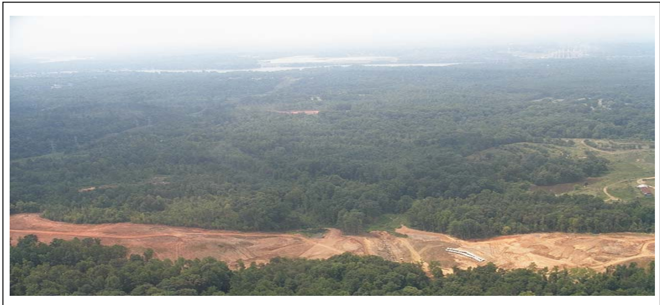
Looking west toward the Catawba River. A view of land cleared for Interstate I-485.
