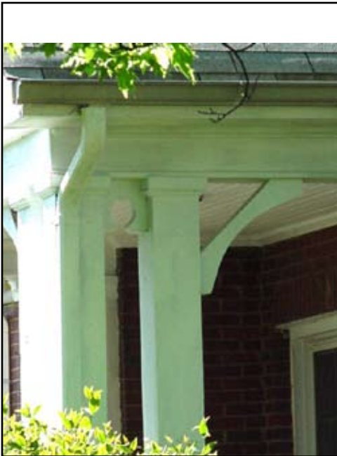
• Downspouts are located appropriately and gutters do not alter or obscure trim.
