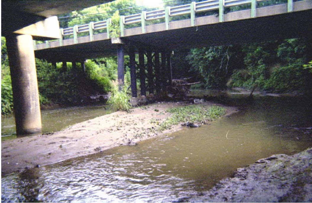
Sugar Creek View, U/S Roll #5 Photo #18 DOWNSTREAM FACE OF ARROWOOD ROAD BRIDGE (WEST BOUND). EROSION AROUND PIERS ON THE RIGHT SIDE (LOOKING DOWNSTREAM).
