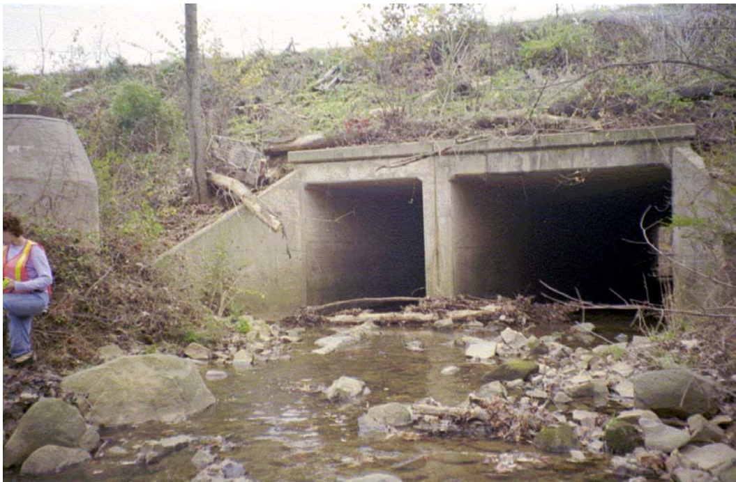
Taggart Creek View, U/S FACE Roll #2 Photo #23 UPSTREAM FACE OF DOUBLE BARREL BOX CULVERT UNDER WILKINSON BLVD. BOULDERS IN CHANNEL WITH SANDY-SILTLY BOTTOM. SOME MILD LOWER BANK EROSION.
