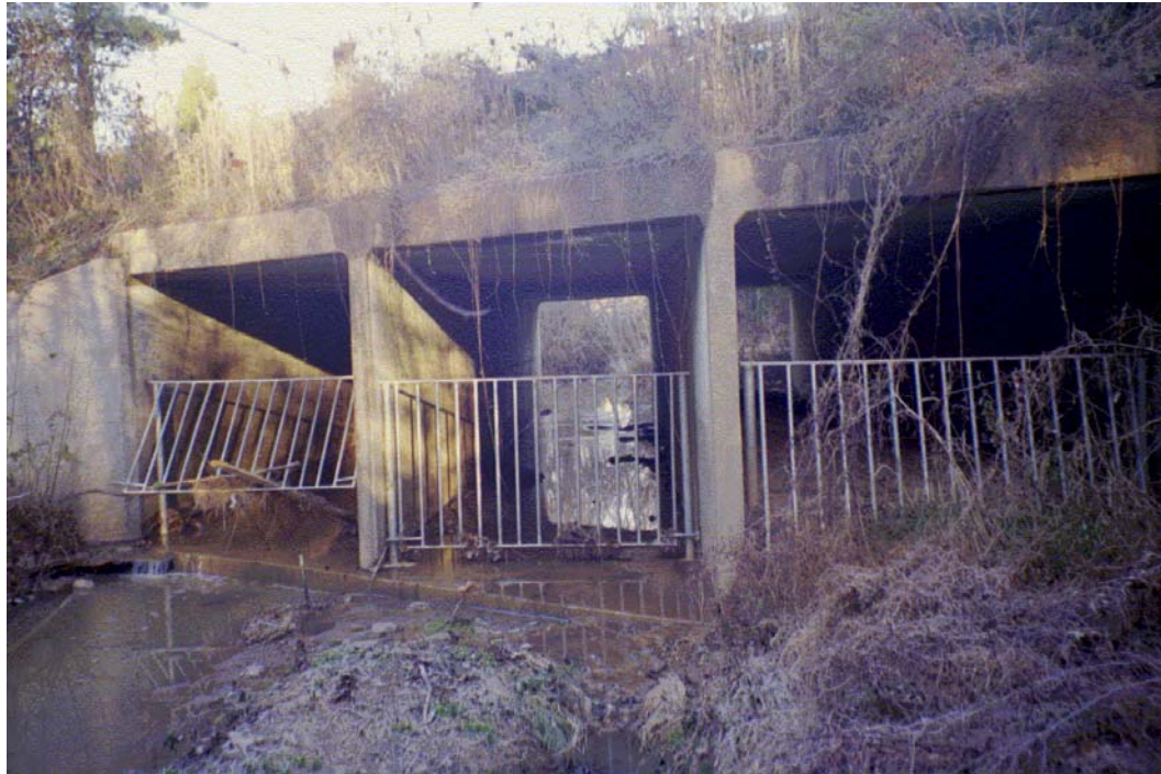
Coffey Creek View, D/S Face Roll #1 Photo #1 LOOKING AT D/S FACE OF WEST BLVD, TRASH RACKS ACROSS THREE BOX CULVERTS. ONE BOX HAS 2.5 FT OF DEPOSITED SEDIMENT.
