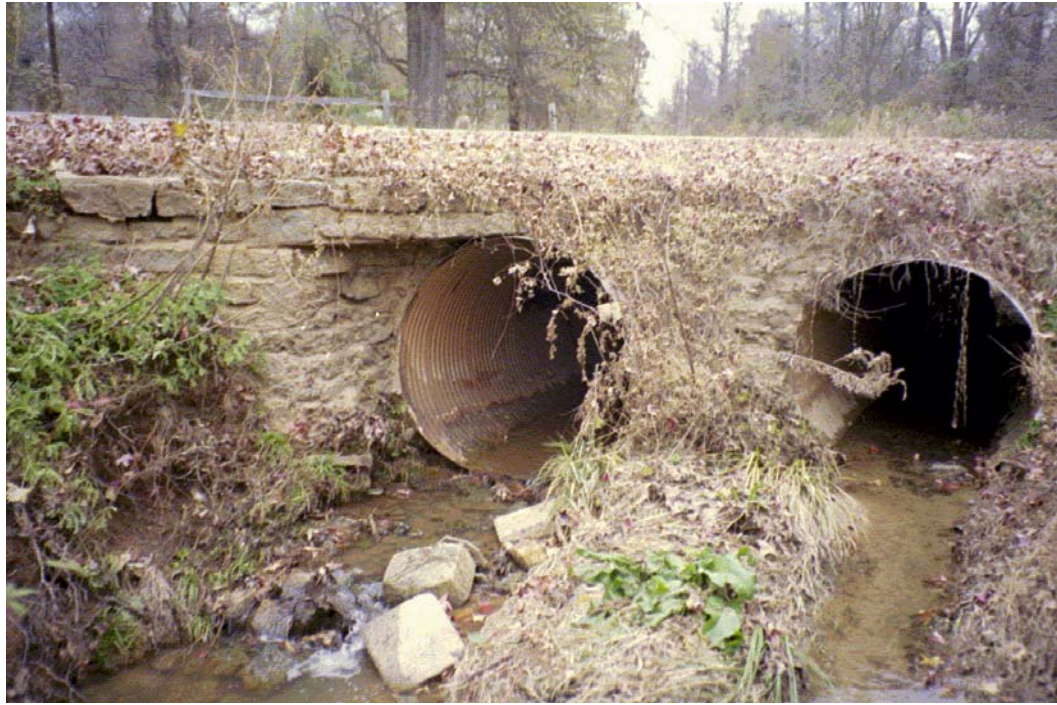
Taggart Creek View, D/S FACE Roll #2 Photo #24 DOWNSTREAM FACE OF DOUBLE BARREL CULVERT UNDER DENVER AVENUE. UPSTREAM AREA IS HEAVILY FORESTED.
