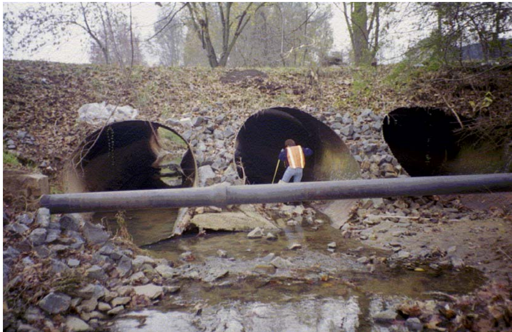
Kings Branch View, U/S Face Roll #1 Photo #22 UPSTREAM FACE OF ARCHDALE DRIVE CROSSING. SANITARY SEWER CROSSING 3.5 FEET ABOVE STREAM.
