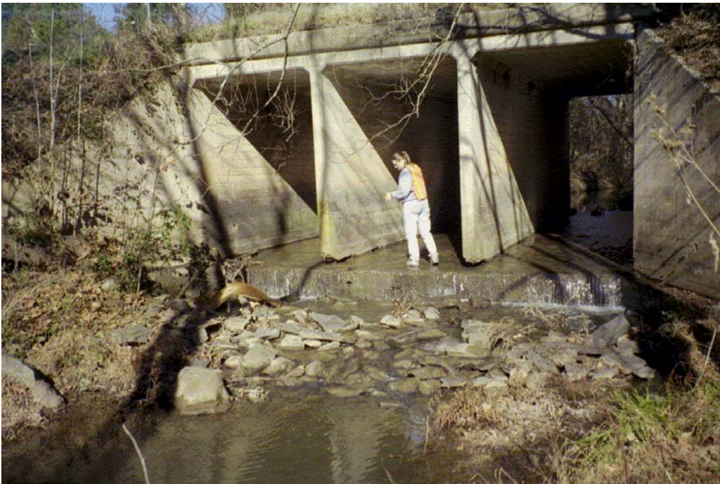
McCullough Creek View, D/S FACE Roll #1 Photo #18 DOWNSTREAM FACE OF THREE BARREL BOX CULVERT UNDER US 51. EVIDENCE OF HEADCUTTING. STABLE BANKS WITH RIPARIAN VEGETATION.
