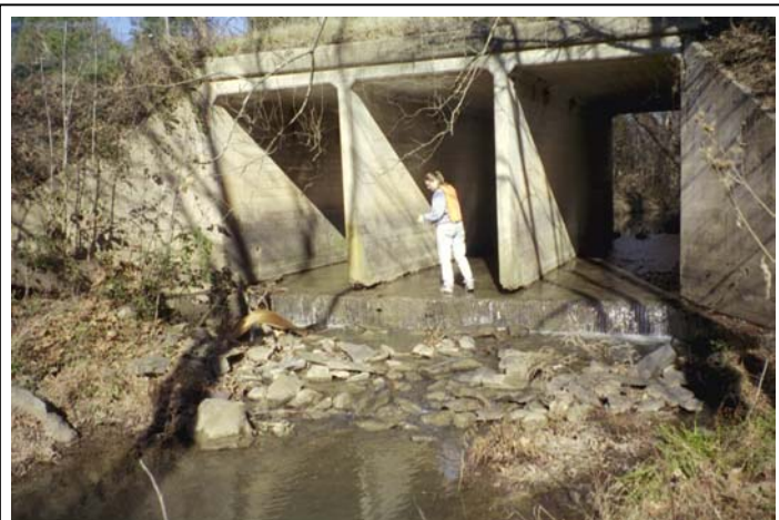
Figure 9. Headcutting on McCullough Creek at Highway 51, Looking at Downstream Face (Roll #1, Photo #18)
