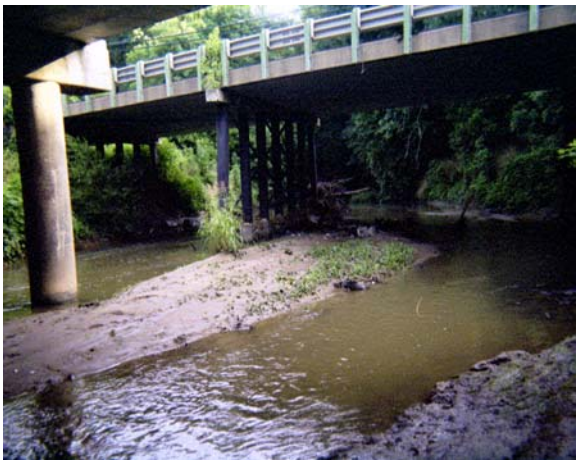
Figure 13. Pier Scouring, Sugar Creek on Westbound Bridge of W. Arrowood Road (Roll #5, Photo #18)
