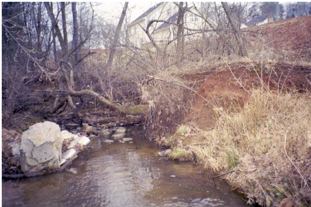
Clarks Creek View, D/S Roll #1 Photo #3 EROSION OBSERVED ON RIGHT BANK, LOOKING DOWNSTREAM OF DEARMON ROAD CROSSING.
