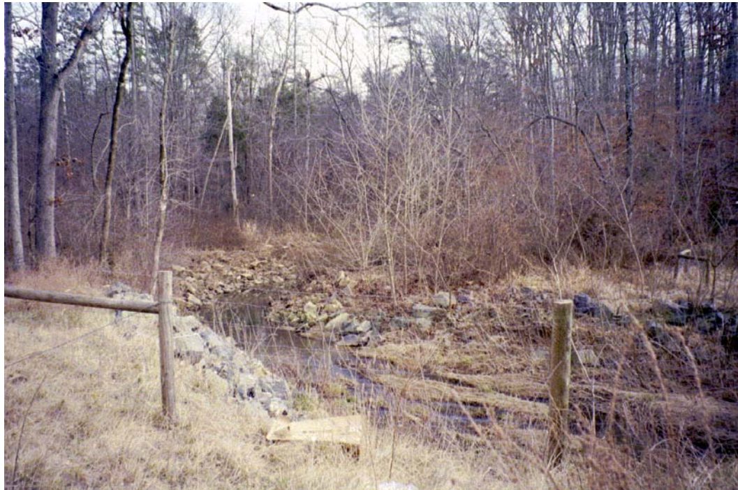
Stoney Creek View D/S Roll #2 Photo #11 DOWNSTREAM OF I-485 BOX CULVERT CROSSING. BANKS STABILIZED WITH RIPRAP.
