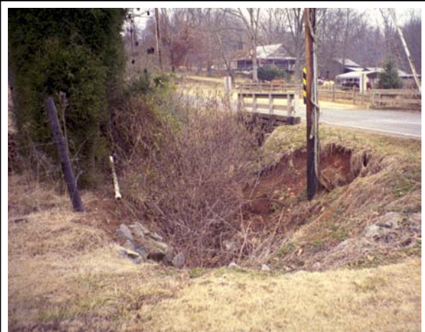
Figure 15. Erosion, Clarks Creek Tributary No. 1 at Hucks Road (Roll #1, Photo #8)
