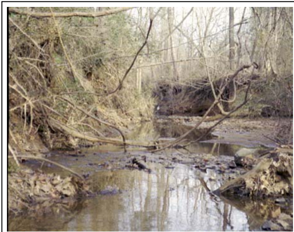
Figure 18. Bank Erosion, Toby Creek at Rocky River Rd, View Downstream. (Roll #3 Photo#13)
