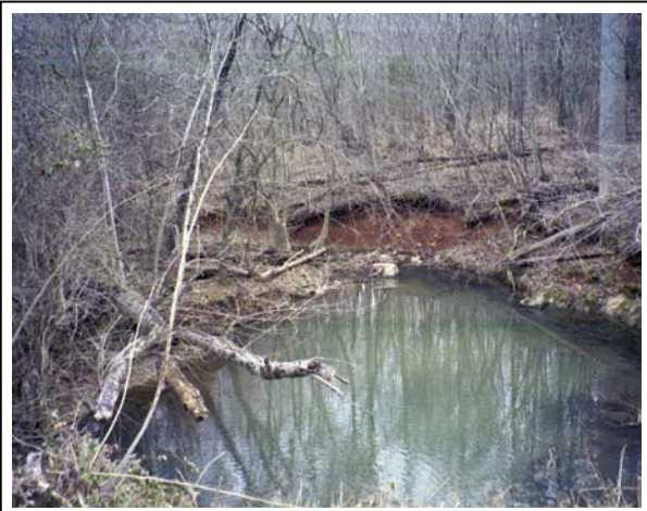
Figure 19. Bank Erosion, Stoney Creek Downstream of Homewood Drive. (Roll #2 Photo #15)
