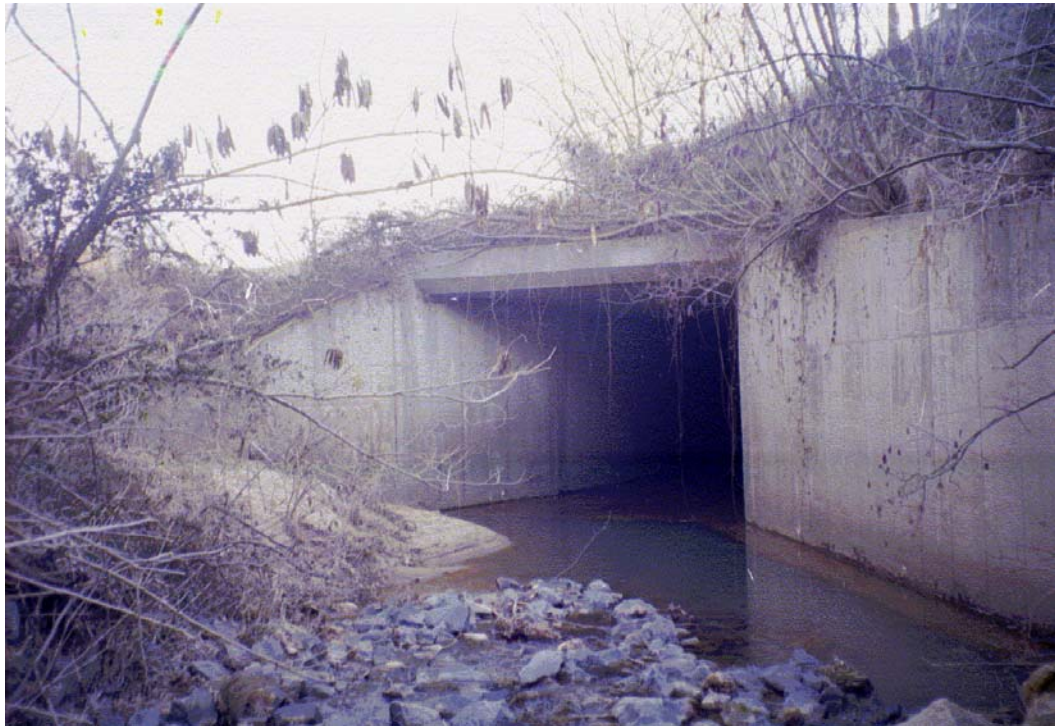
Doby Creek View U/S Roll #2 Photo #24 UPSTREAM FACE OF 12'x11' CONCRETE BOX CULVERT CROSSING W.T. HARRIS BOULEVARD. BOX CULVERT BENDS UNDER ROAD.
