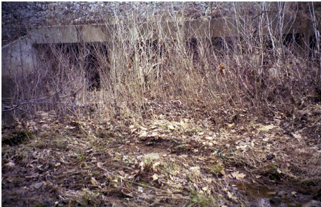
Mallard Creek View, U/S Roll #1 EXTENSIVE DEPOSITION IN UPSTREAM FACE OF 4 BARREL 13' x 9' BOX CULVERT CROSSING AT W.T. HARRIS BOULEVARD.
