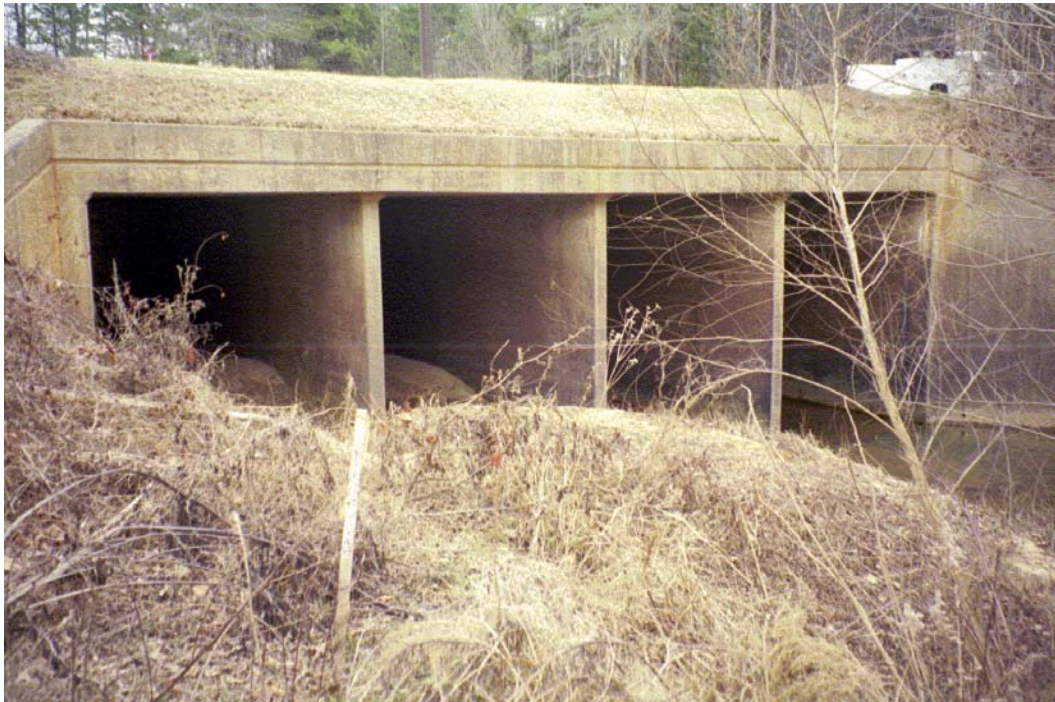
Mallard Creek View, U/S Roll #1 Photo #22 SCOUR ON UPSTREAM FACE OF 4 BARREL 12' x 15' CONCRETE BOX CULVERT CROSSING AT DAVID TAYLOR DRIVE. SEDIMENT DEPOSITED IN 3 BARRELS OF CROSSING.
