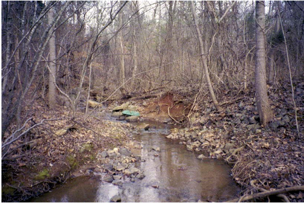
Doby Creek Tributary # 1 View D/S Roll #2 Photo #18 RIGHTBANK EROSION DOWNSTREAM OF IBM DRIVE (UPPER) CULVERT CROSSING.
