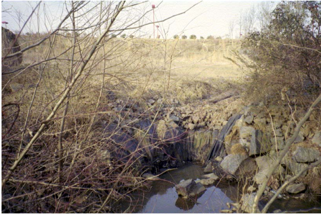
Toby Creek View D/S Roll #3 Photo #9 DRAINAGE ON LEFT BANK NEAR CHANCELLORS PARK CULVERT CROSSING. HEAD CUTTING PREVENTION MEASURES PRESENT.
