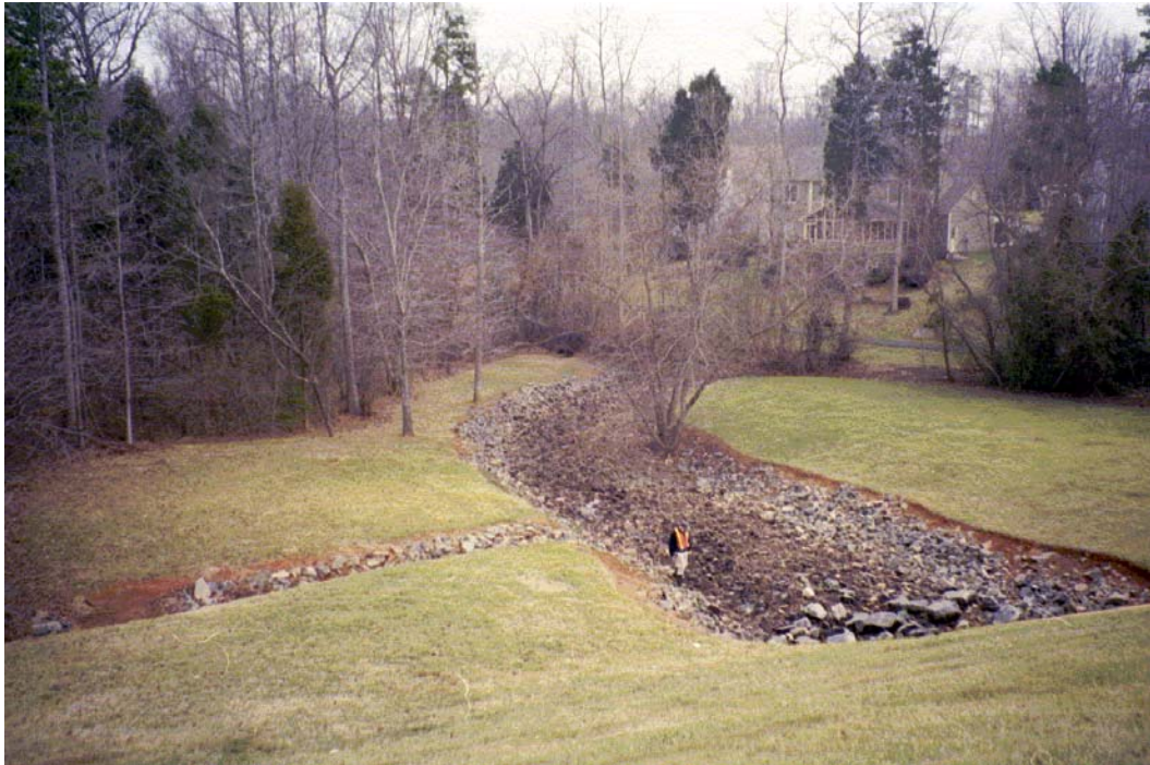
Clarks Creek Tributary #1A View, D/S RIPRAP CHANNEL DOWNSTREAM OF DAVIS LAKE OUTLET STRUCTURE. MOWING TO EDGE OF STREAM CHANNEL.
