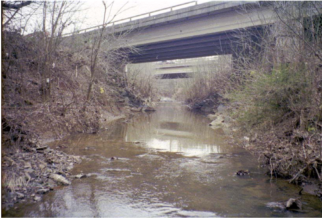
Mallard Creek View, D/S Roll #1 Photo #24 DOWNSTREAM FACE OF 2 BRIDGE CROSSINGS AT I-85. ENTRENCHED, STRAIGHT CHANNEL.
