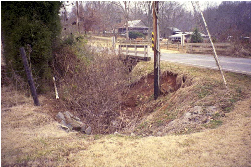
Clarks Creek Tributary #1 View, D/S Roll #1 EROSION OBSERVED AT DOWNSTREAM SIDE OF HUCKS ROAD CROSSING. CITY WATER MAIN FLUSHED WEEKLY INTO DRAINAGE CHANNEL.
