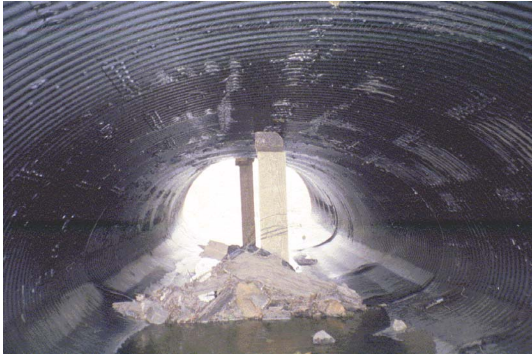
Stoney Creek View inside culvert Roll #2 Photo #16 INSIDE OF 12' x 7.5' CMPA AT MALLARD CREEK ROAD. CULVERT IS COLLAPSING AND CURRENTLY SUPPORTED BY PILLARS. DEBRIS IS COLLECTING INSIDE CULVERT.
