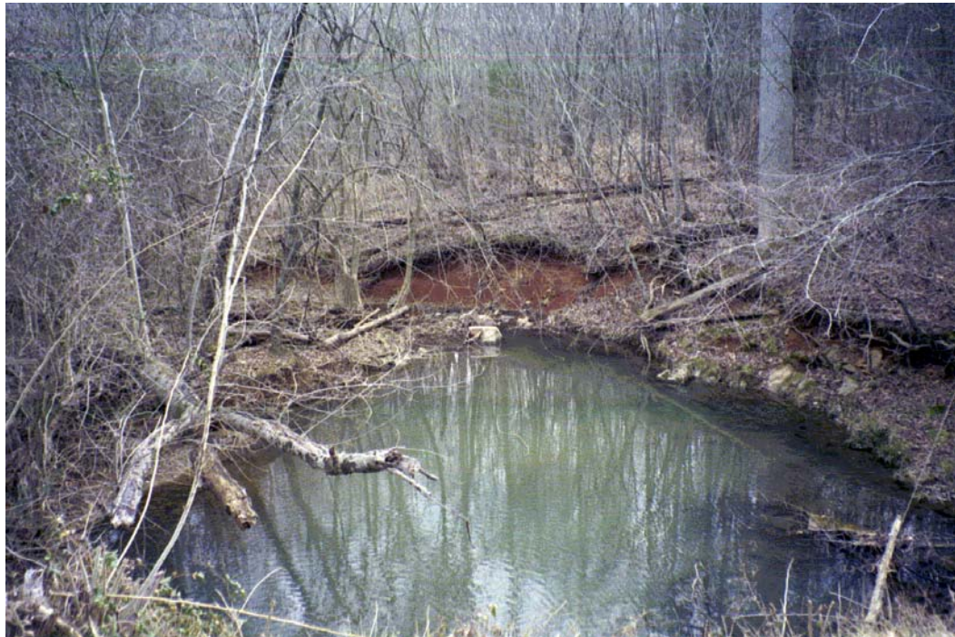
Stoney Creek Tributary View D/S Roll #2 Photo #15 LARGE POOL AND ERODED RIGHT BANK (LOOKING DOWNSTREAM) OF HOMEWOOD DRIVE CULVERT CROSSING.
