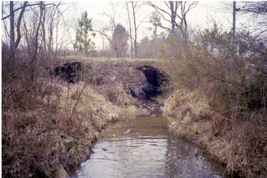
Clarks Creek View, D/S Roll #1 Photo #2 DOWNSTREAM FACE OF 3 BARRELCMPA 102"x72" CROSSING AT DEARMON RD.
