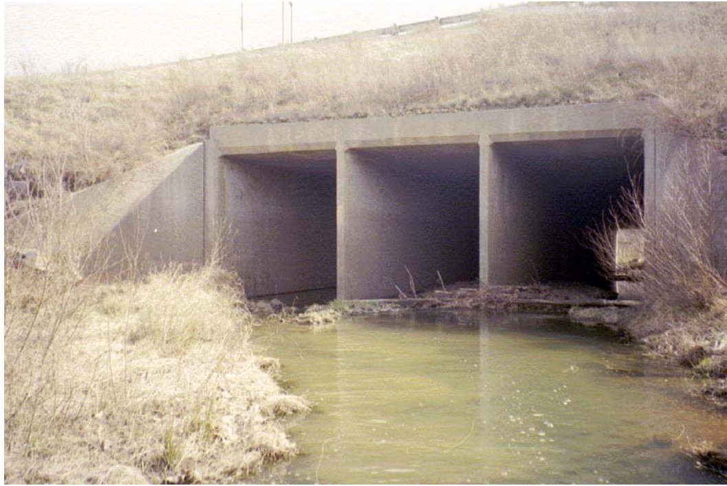
Stoney Creek View, U/S Roll #2 Photo #10 UPSTREAM FACE OF 3 BARREL 11' x 13' CONCRETE BOX CULVERT CROSSING AT US 29/TRYON STREET. COBBLES HAVE ACCUMULATED IN RIGHT 2 BARRELS.
