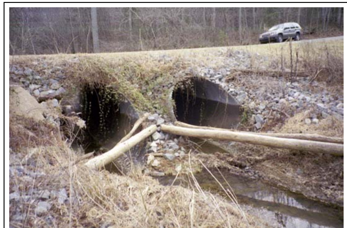
Figure 7. Typical Channel, Stoney Creek Tributary at Homewood Drive, Looking at Upstream Face (Roll #2, Photo #14)
