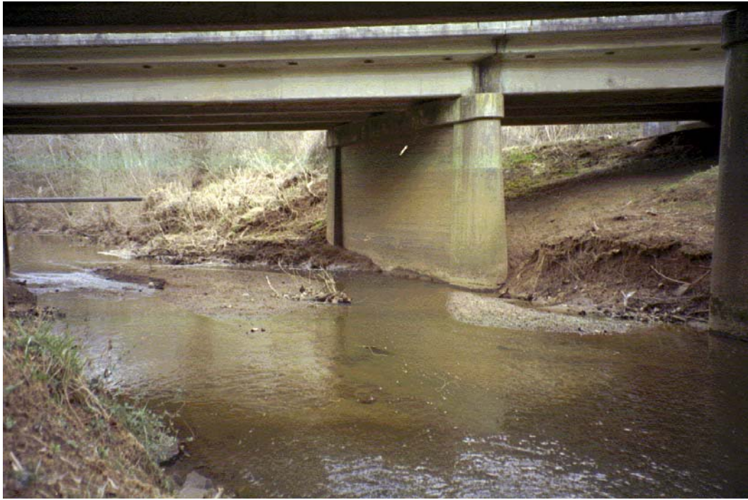
Mallard Creek View, D/S Roll #2 Photo #4 LOWER BANK EROSION AT N. TRYON STREET. SANITARY SEWER CROSSING IN BACKGROUND.
