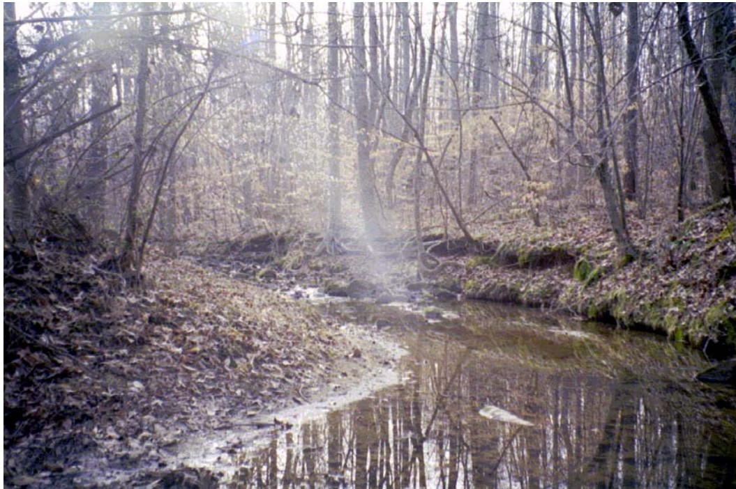
Toby Creek View U/S Roll #3 MILD BANK EROSION UPSTREAM OF AUTUMNWOOD CT. CULVERT CROSSING.
