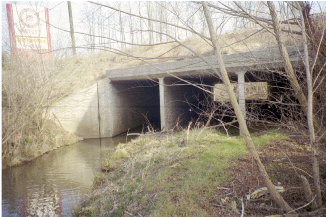
Toby Creek View U/S Roll #3 Photo #8 UPSTREAM FACE OF 5 BARREL 10' x 10' CONCRETE BOX CULVERT CROSSING CHANCELLORS PARK. DEPOSITION PRESENT IN 4 BARRELS.
