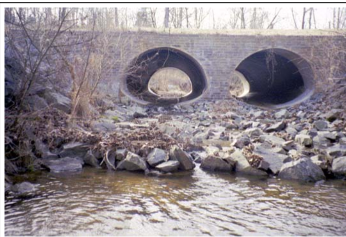
Figure 13. Riprap Stabilization, Toby Creek at Rocky River Road Looking at Downstream Face (Roll #3, Photo #12)
