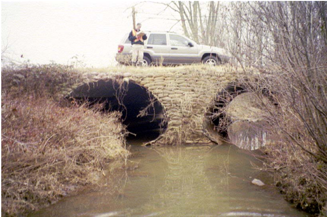
Clarks Creek Tributary #1 View, U/S Roll #1 Photo #10 UPSTREAM FACE OF DOUBLE BARREL CMPA CROSSING AT BROWNE ROAD.
