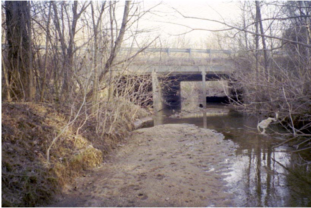
Toby Creek View U/S Roll #3 Photo #3 UPSTREAM FACE OF 3 BARREL 10'x 9' BOX CULVERT CROSSING AT TOBY CREEK ROAD. DEPOSITION PRESENT AT UPSTREAM SIDE, DOWNCUTTING OCCURRING DOWNSTREAM.
