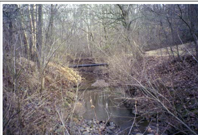
Figure 10. Sanitary Sewer Line Crossing Doby Creek Tributary (Roll #2, Photo #20)
