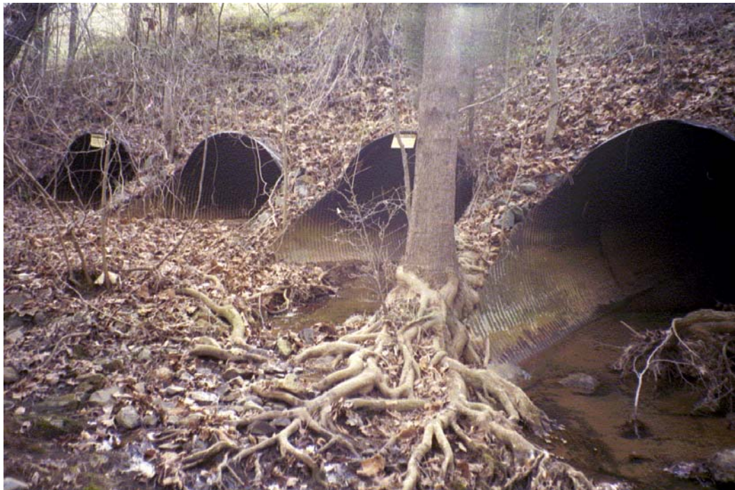
Doby Creek Tributary # 1 View D/S Roll #2 Photo #19 DOWNSTREAM FACE OF 5 BARRELS 7' 10" CMP CROSSING AT IBM DRIVE (UPPER). SEDIMENT PRESENT IN 2 LEFT BARRELS.
