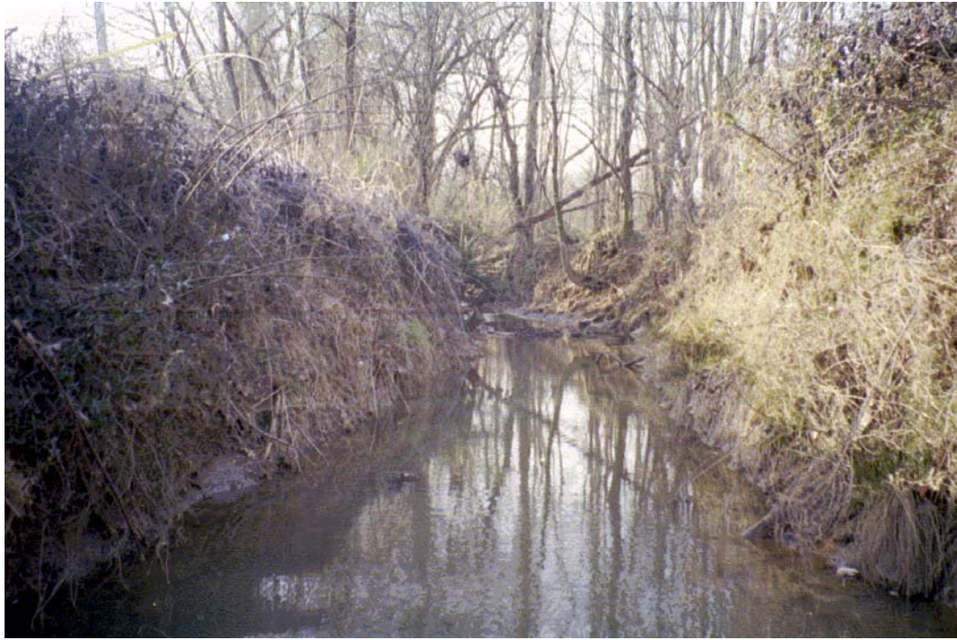
Toby Creek View U/S Roll #3 Photo #6 SEVERE DOWNCUTTING UPSTREAM OF CONCRETE BOX CULVERT CROSSING HWY 49. OBSERVED BEAVER.
