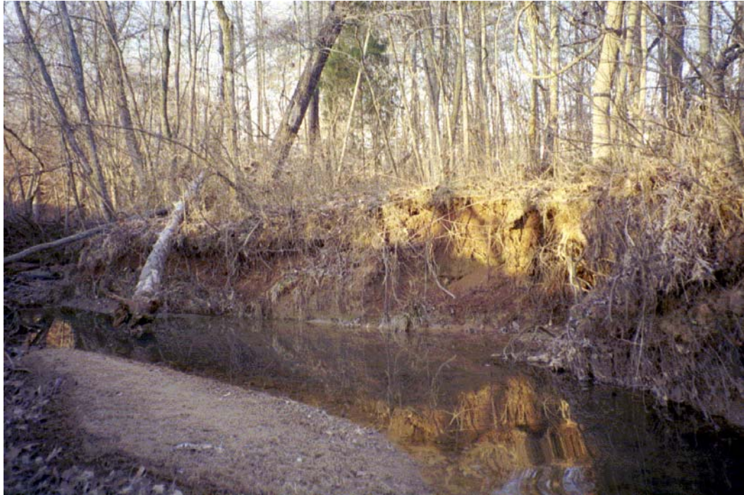
Doby Creek View U/S Roll #2 Photo # 22 BANK EROSION UPSTREAM OF GOVERNOR HUNT MIDDLE SCHOOL ROAD CONCRETE BRIDGE CROSSING.
