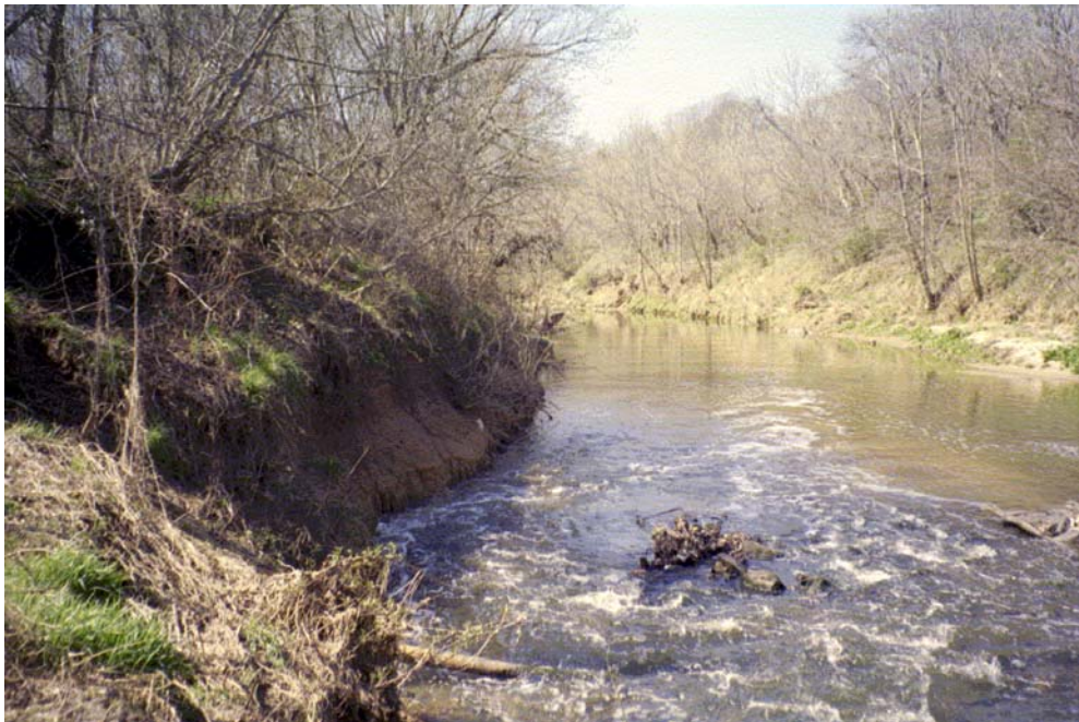
Lower Little Sugar Creek View D/S Roll #4 Photo #21 RIFFLS DOWNSTREAM OF POLK ROAD BRIDGE CROSSING. LOWER LEFT BANK EROSION. TOE IS UNPROTECTED.
