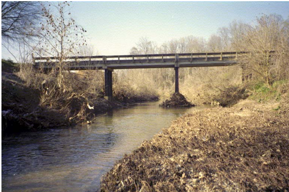
Lower Little Sugar Creek View U/S Roll #4 Photo #5 UPSTREAM FACE OF BRIDGE CROSSING TO WWTP. SAND DEPOSITION AND DEBRIS ACCUMULATION. SCOUR PRESENT ON CENTER PIER.
