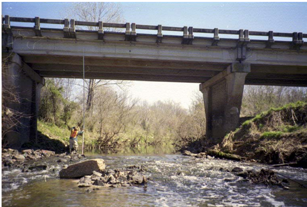
Lower Little Sugar Creek View D/S Roll #4 Photo #23 DOWNSTREAM FACE OF POLK ROAD BRIDGE CROSSING.
