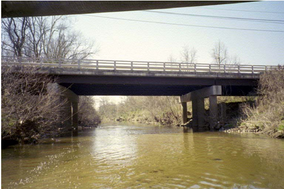
Lower Little Sugar Creek View D/S Roll #4 Photo #14 SHALLOW FLOW DOWNSTREAM OF SHARON ROAD WEST BRIDGE CROSSING.
