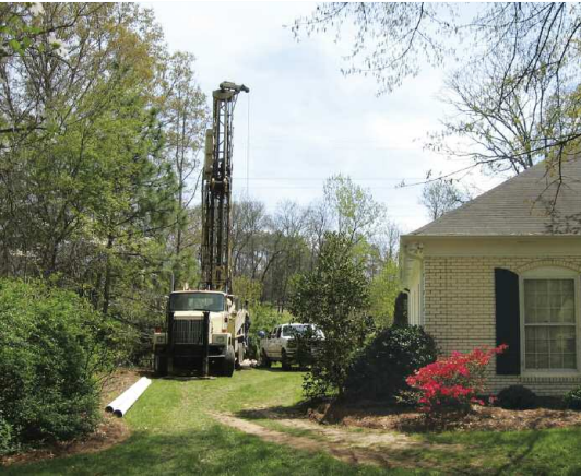
20-foot sections of 6-inch diameter PVC casing lying on the ground in front of an operating drill rig.
