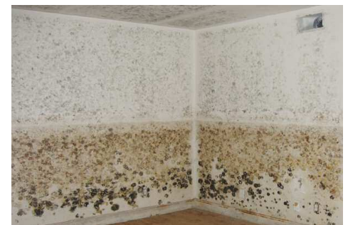
Mold growth after residential flood.
