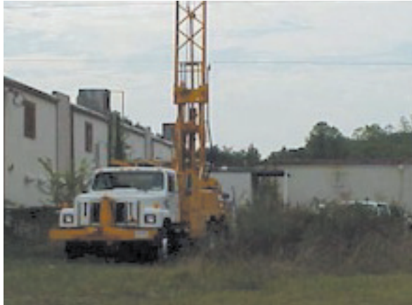
EPA Team investigating the extent of contamination at a drycleaning facility.
