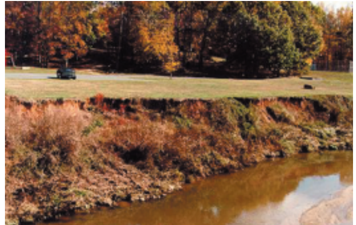
Mecklenburg County Storm Water Services Little Sugar Creek streambank stabilization project combined hard engineering techniques (rip-rap) and soil bioengineering to stabilize the streambank.
