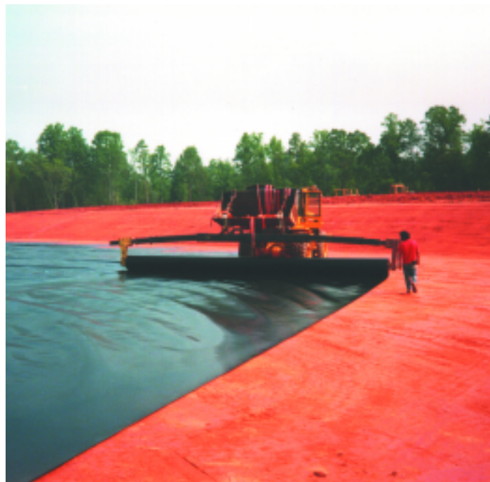
Workers install the plastic membrane of the landfill's composite liner system. The plastic covers three feet of clay and is itself covered by the leachate collection system and a top covering of dirt.
