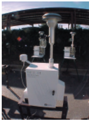
Typical PM 2.5 particulate monitor.
