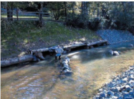
Fish lunkers, or constructed bank overhangs, installed in Briar Creek provide cover and refuge for fish.
