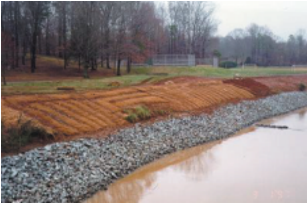
2 years after construction, the vegetation has stabilized Little Sugar Creek's streambank in Huntingtowne Farms Park.
