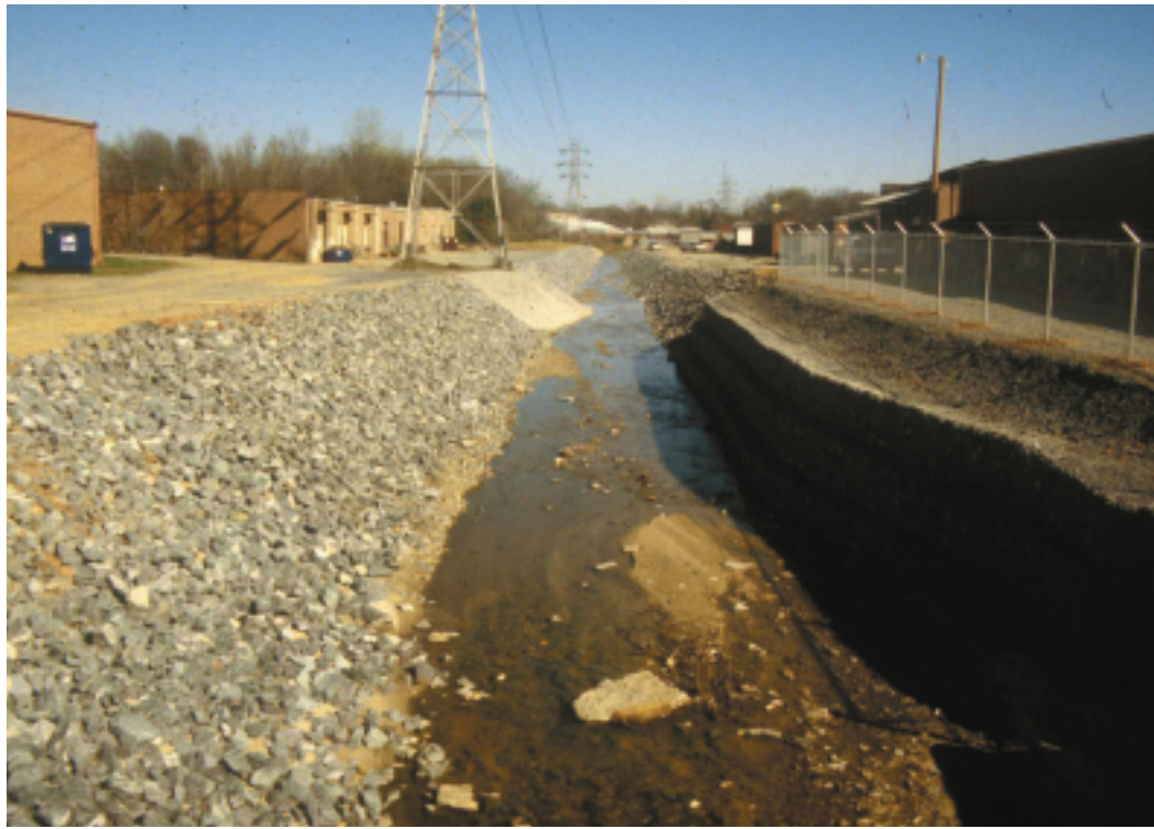
This straight section of Little Sugar Creek near E. 36th Street is typical of past engineering designs to control streambank erosion and flooding.
