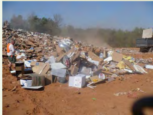
Photo 6.1 Construction & Demolition Debris
