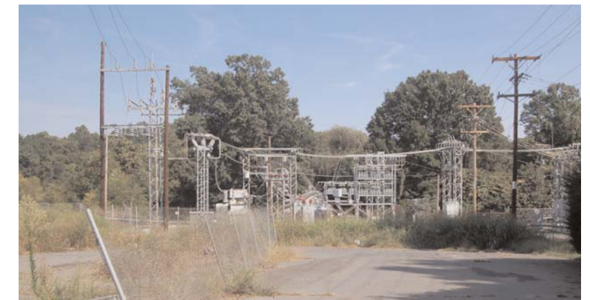
EXISTING CONDITIONS Electrical sub station north of Third Street
