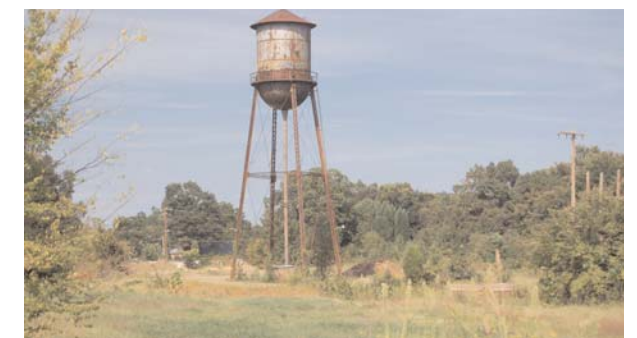
EXISTING CONDITIONS Abandoned water tower on the Anchor Mill Site that could become an iconic symbol for the new development
