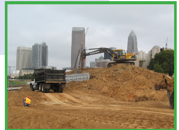
Construction is currently underway on I-277 ramps and surrounding streets as part of the I-277/Caldwell Interchange Project (NASCAR Hall of Fame Road Improvements).
